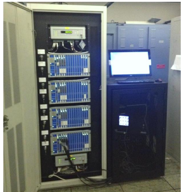
Figure 1 – Workstation half-height cabinet containing SETPOINT pilot system (right) and Bently Nevada 3500 series racks (left). 3500 rack #4 (bottom-most) is for the compressor train; rack #3 (second from bottom) is for the pump train.
